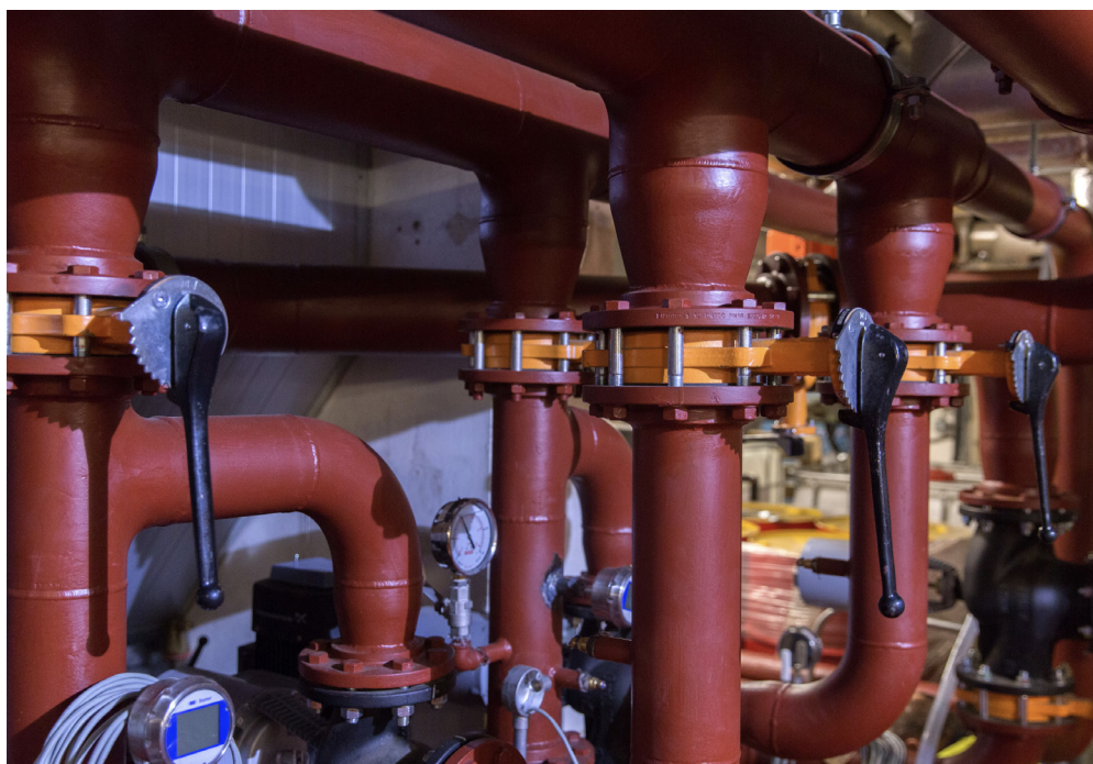
Pipework in the combined heat and power plant
