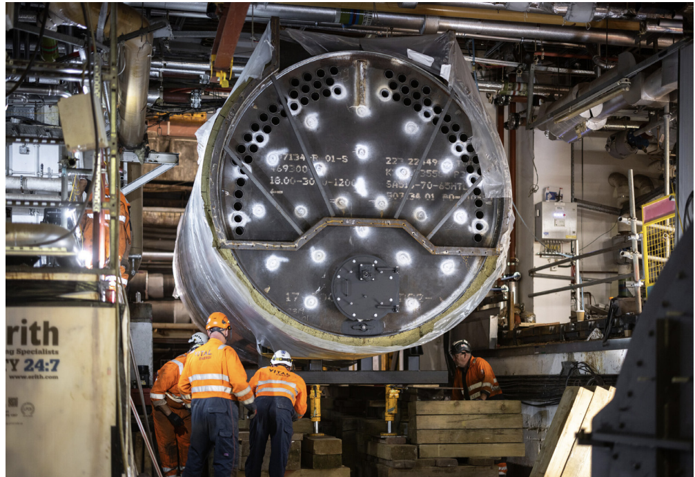
One of the three new boilers being installed in the energy centre
